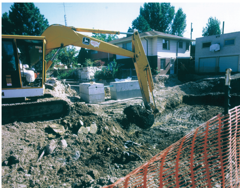
FIGURE 7.2 Excavation of uranium mill tailings from a residential septic system, Grand Junction, Colorado, 1993. SOURCE: USDOE Office of Environmental Management.
